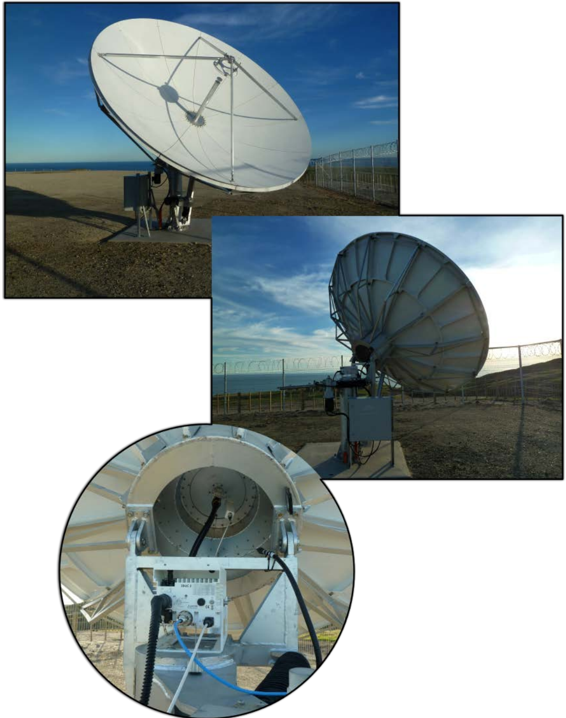
Figure 3.2 IBUC 2 Field Installation
