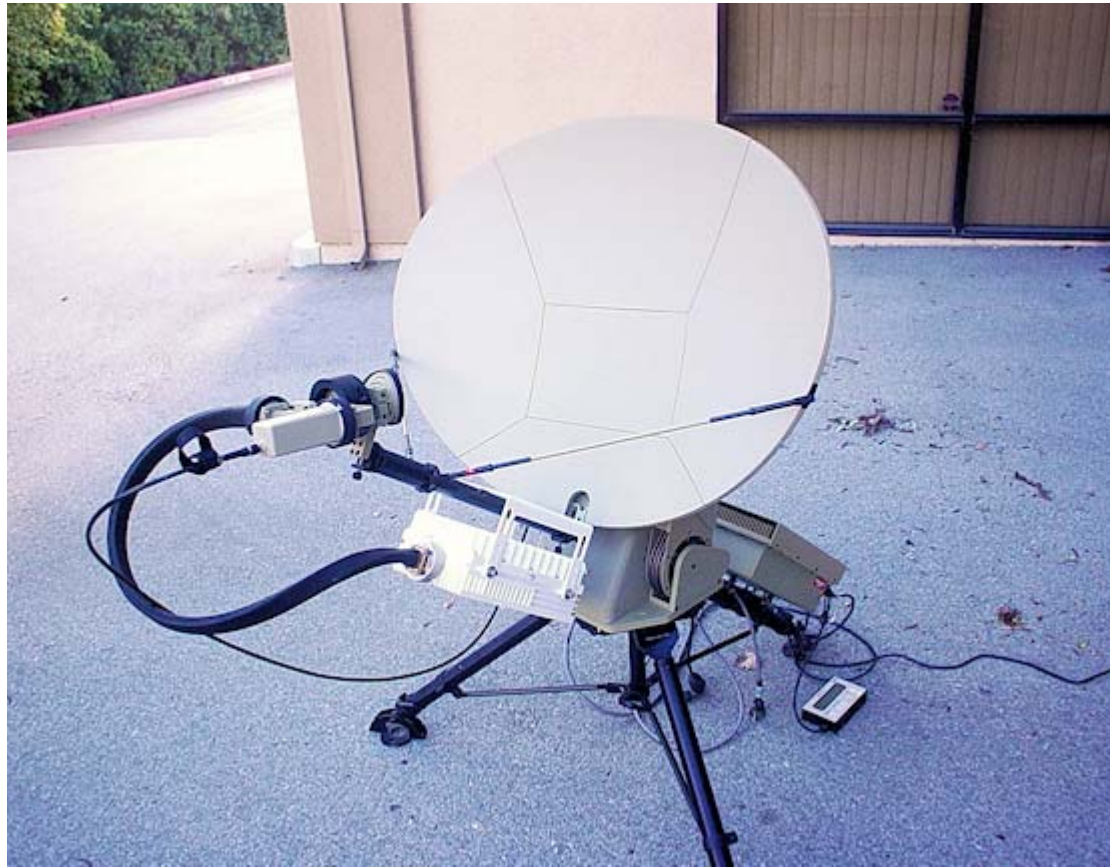
Figure 3.2 IBUC 2 Field Installation
