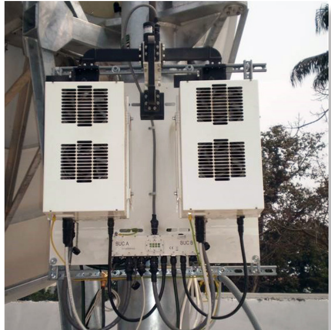
Field installation of Redundant IBUCs
